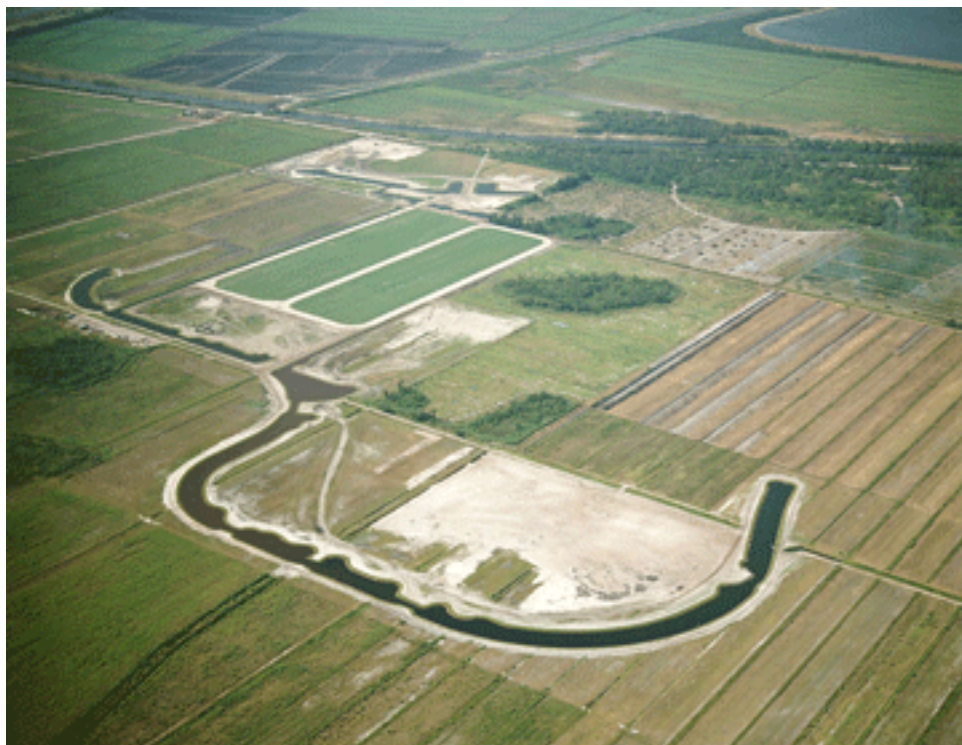
Aerial view of the Lake Point Project showing the progress in heavy ground work including the four polo fields at the center of phase I.
